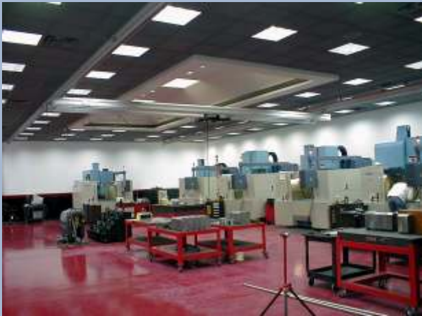
A ceiling mounted double girder system moves machined parts among workstations. Runway supports are mounted above ceiling tiles for a clean, uncluttered appearance.
